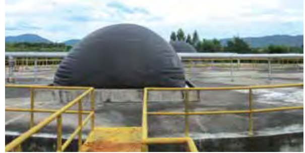
Biogas plant at Cholcharoen cassava starch factory.
