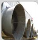
Evaporative Cooling System (Evap)
